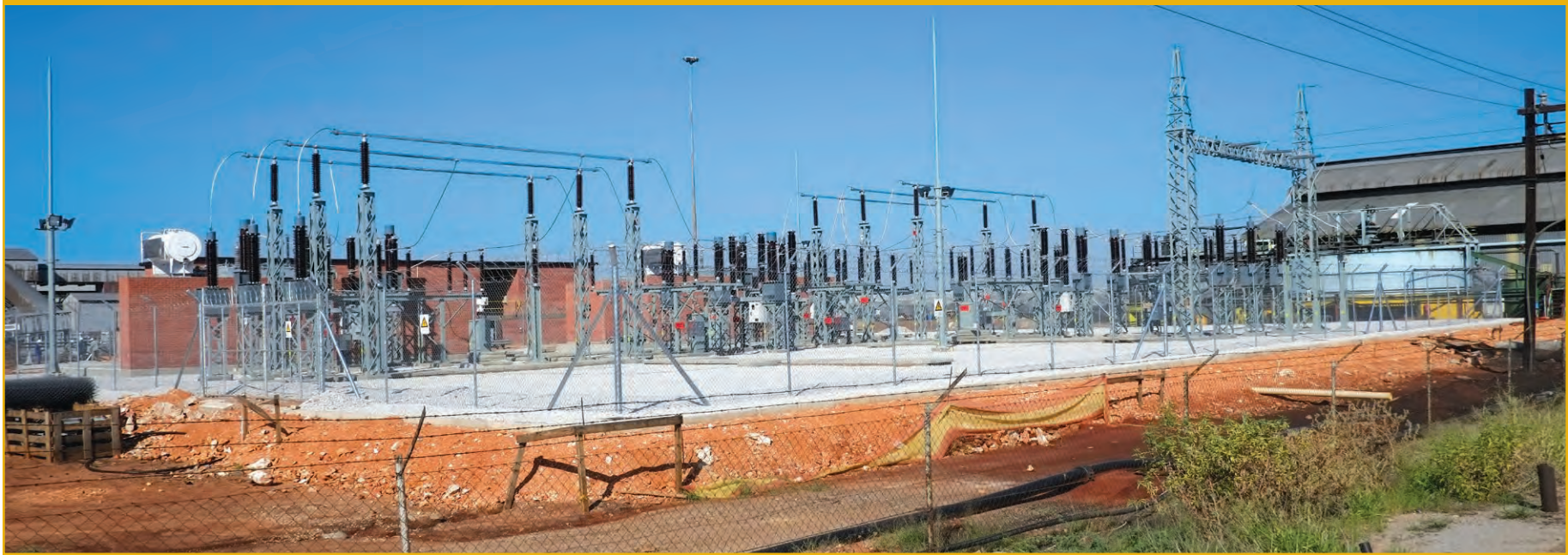
Power substation, Tsumeb
